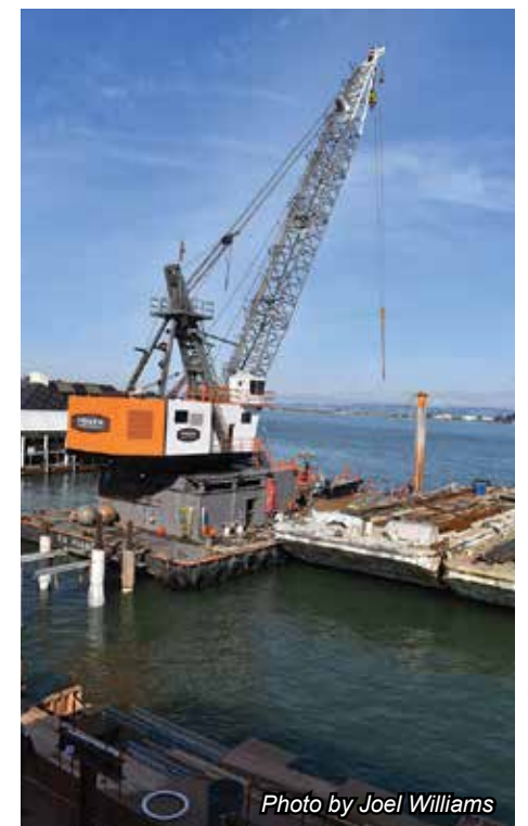
Construction materials and debris are being delivered and removed by barge in order to keep traffic and roadways on Embarcadero clear.
