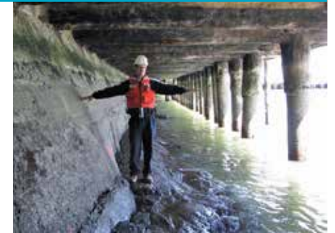
A major earthquake could cause the seawall to be pushed forward into the Bay as much as a foot in some places—thereby threatening the wall's structural integrity.
