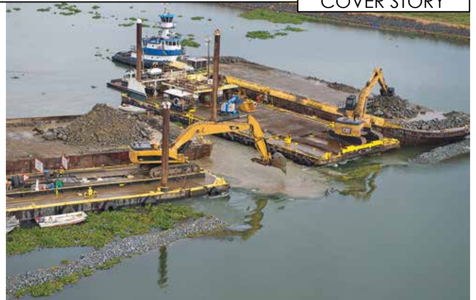
Complete removal of the 750-foot-wide salinity barrier is expected to take 45-60 days and be done by mid-November.
