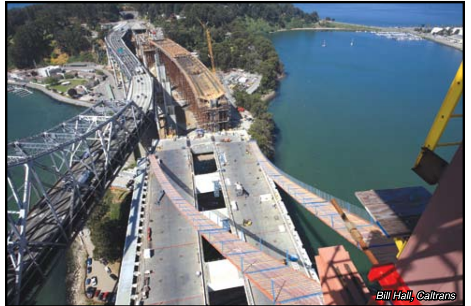
A pair of 600-foot-long catwalks stretch from the East Span tower down to the road decks below.
