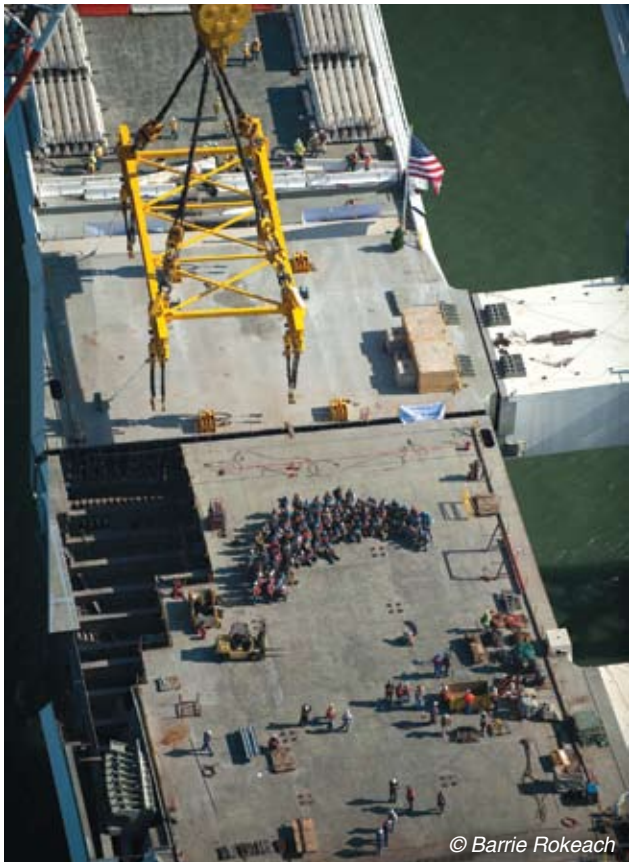
After the operation, the ironworkers gather to mark the completion of the East Span decks.
