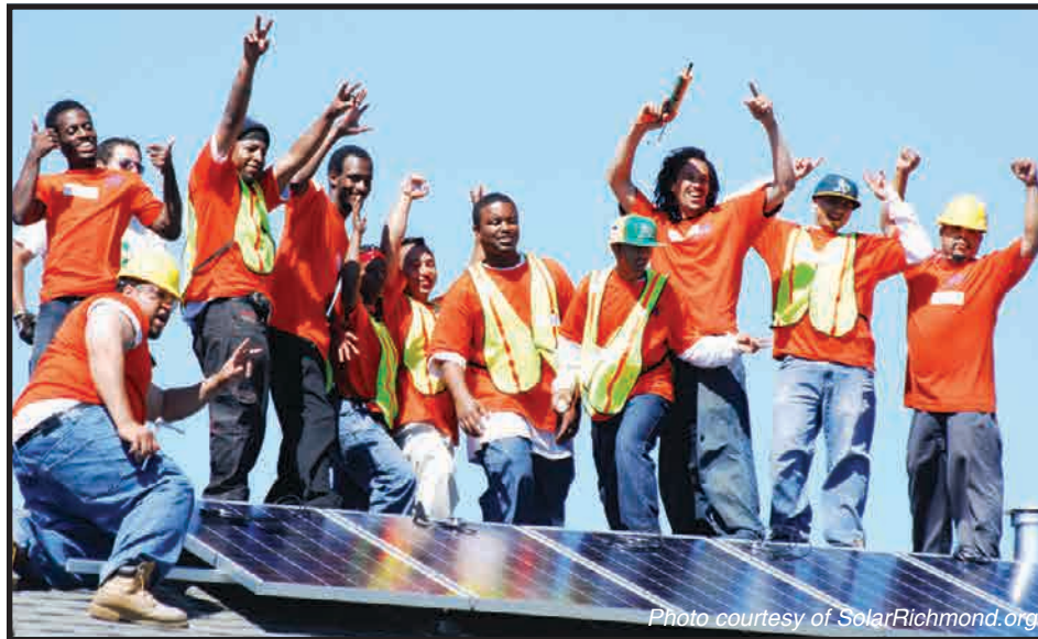
The City of Richmond has partnered with the non-profit organization Solar Richmond to train local youths to install solar panels. This model program has received commendations from both the State and Federal levels.
