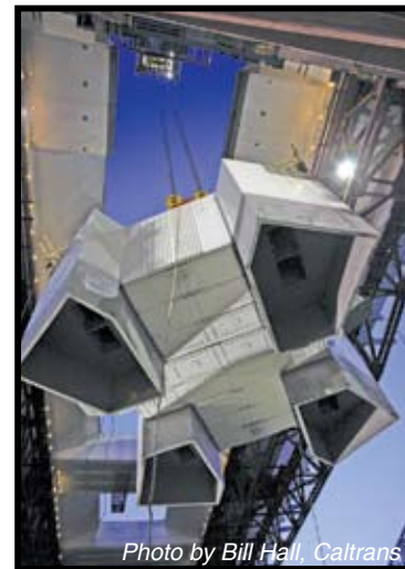
Photo by Bill Hall, Caltrans An underneath view of the grillage piece as it rises between the twin decks of the East Span
