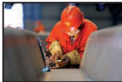
A worker smooths the surface of a “U-rib” that will form part of the new bridge deck.
