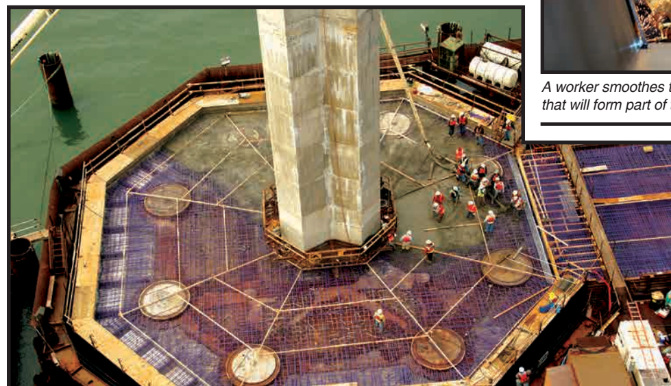
Enormous deep water foundations support the towers that will connect the Skyway section to the Self-Anchored Suspension Span.
