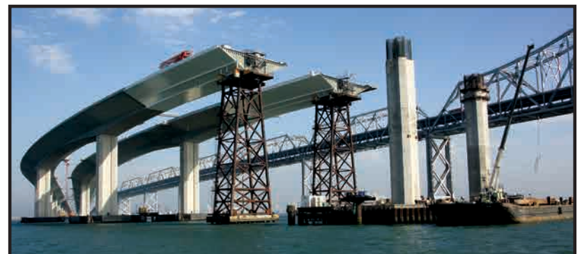
The 1.3-mile Skyway rises gracefully from the East Bay mudflats to a height of 150 feet over San Francisco Bay.
