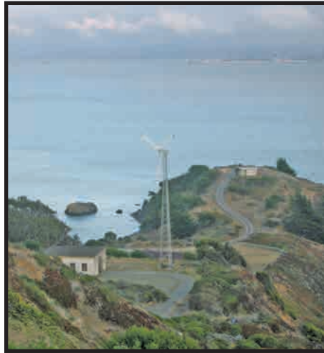
The wind turbine installed 25 years ago on the south side of Angel Island used to provide one-third of the park's electricity.
