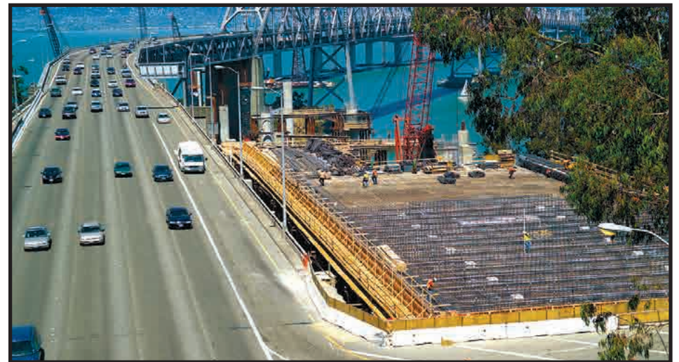
Just east of the Yerba Buena Island tunnel, construction crews are working round-the-clock on a replacement for a key chunk of the upper road deck of the San Francisco-Oakland Bay Bridge. The piece will also function as a link to the tunnel for the new East Span that is now under construction.
