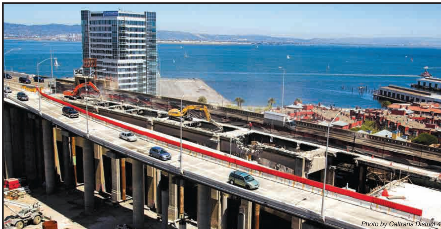
Caltrans crews maintain a delicate balance between creation and destruction to keep traffic moving through downtown San Francisco during the reconstruction of the Bay Bridge West Approach.
